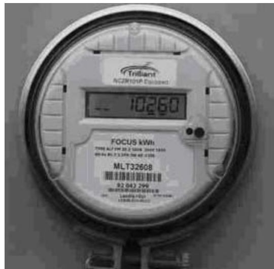
A typical smart meter.
